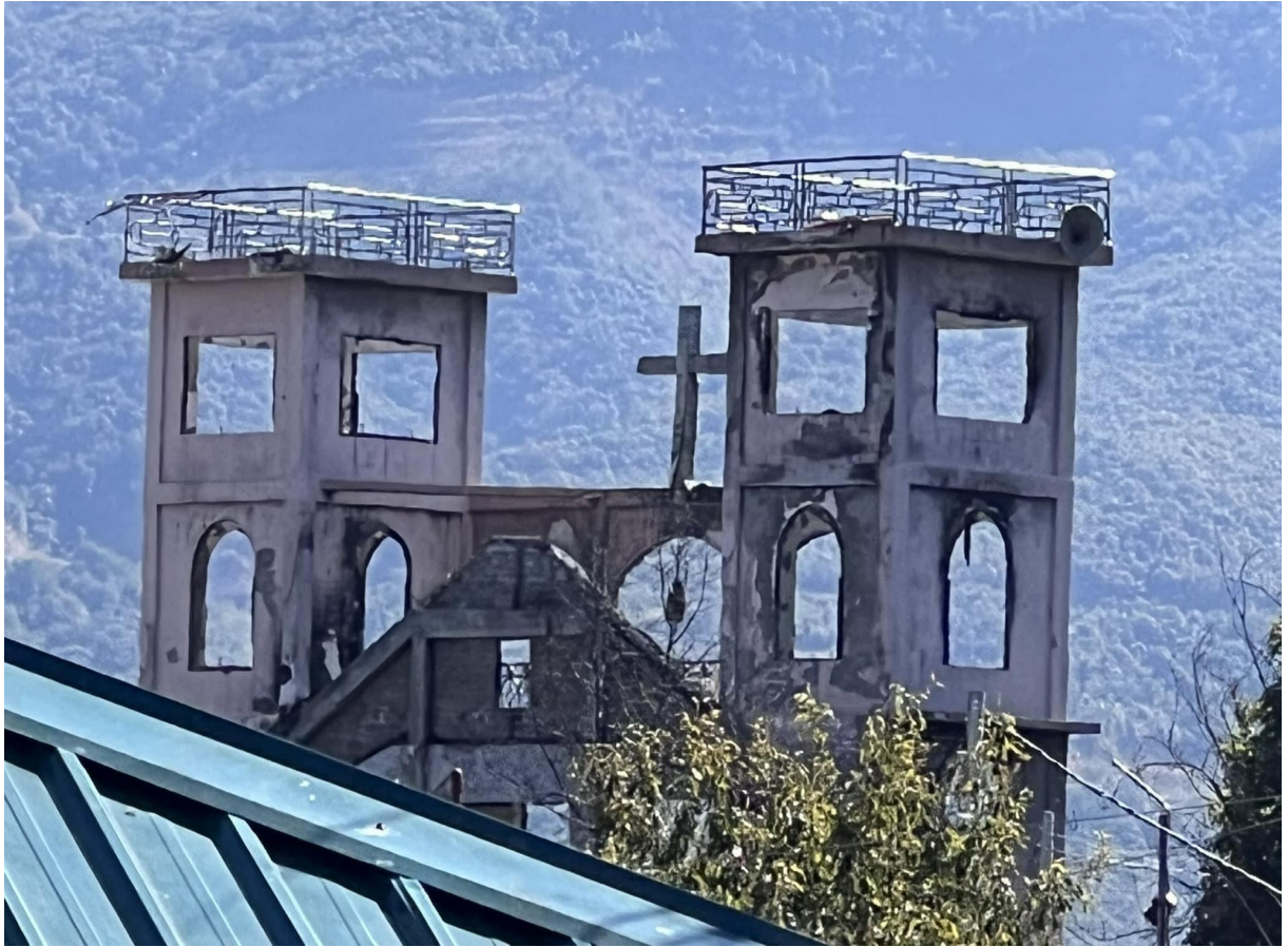
Photograph 12. What remains of the Johnson Memorial Baptist Church after it was completely burned down by the Myanmar military on 24 May 2022.
